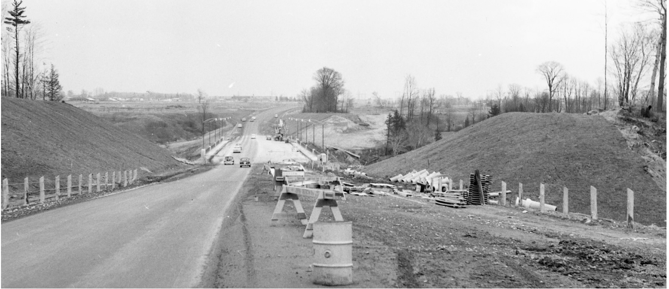
Figure 6: Eglinton Extension under construction in 1956, facing east possibly at Wynford Drive (Toronto Archives).
