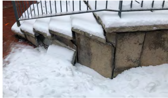
32. Detail of failing stone clad patio (ERA, 2020).
