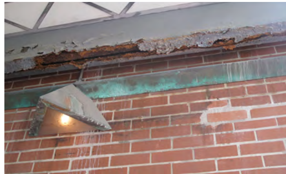
23. Detail of rusted metal canopy (ERA, 2016).
