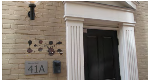
29. In west walkway, detail of single entrance with remnant adhesive and multiple holes from old signage (ERA, 2016).
