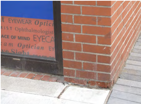
4. Southwest corner, spalled brick at grade (ERA, 2016).
