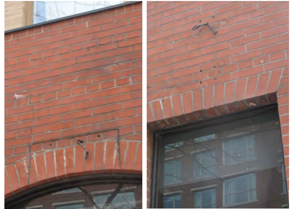
8. Detail of holes, electrical wiring and remnant adhesive from old signage window and door opening (ERA, 2016).
