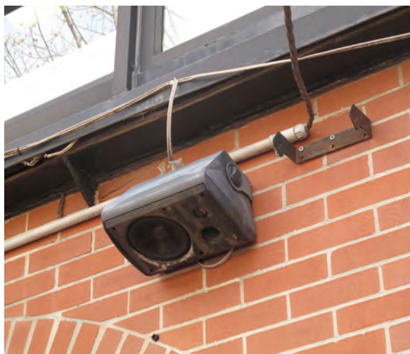
20. Detail of old speaker, speaker hangers and associated wires (ERA, 2016).
