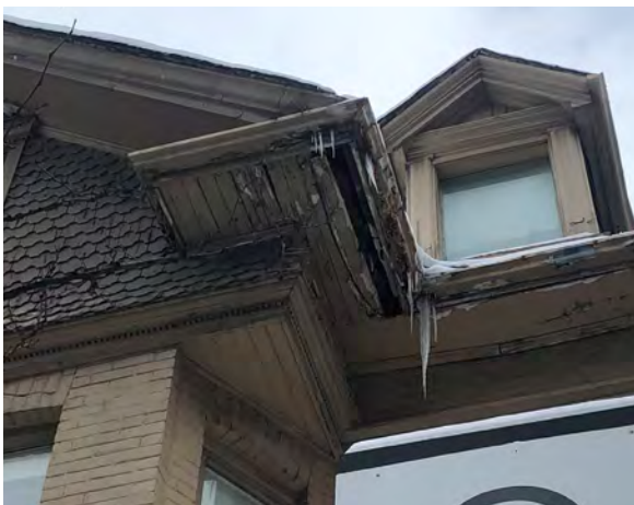
5. Soffit, trim and gutter starting to separate from the roof (ERA, 2020).
