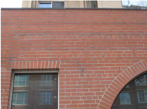
3. Detail showing holes and remnant adhesive from old signage (ERA, 2016).
