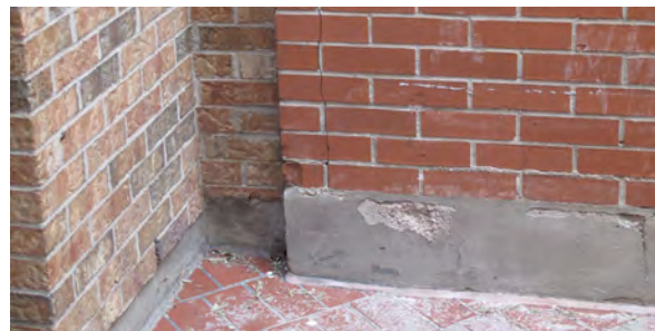
24. Detail of cracks in the brick work chipping of the concrete foundation (ERA, 2016).
