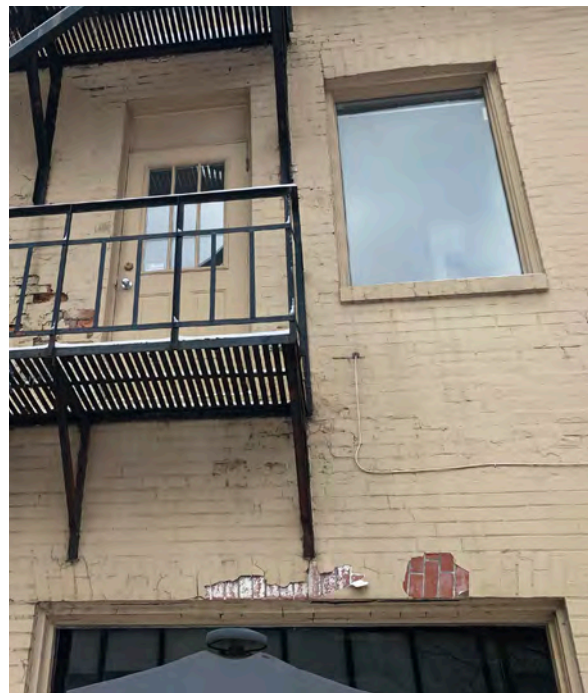
33. Detail paint condition on wall (ERA, 2020).
