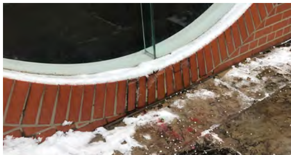
13. Detail of brick spalling on round window, stone veneer and junction between the porch and west facade, above photo dated 2016, below 2020 (ERA, 2016;2020).
