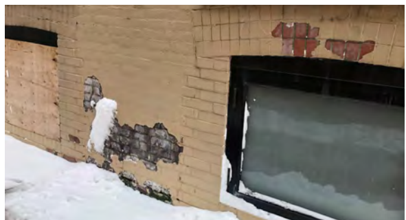
31. Peeling paint in west walkway (ERA, 2020).
