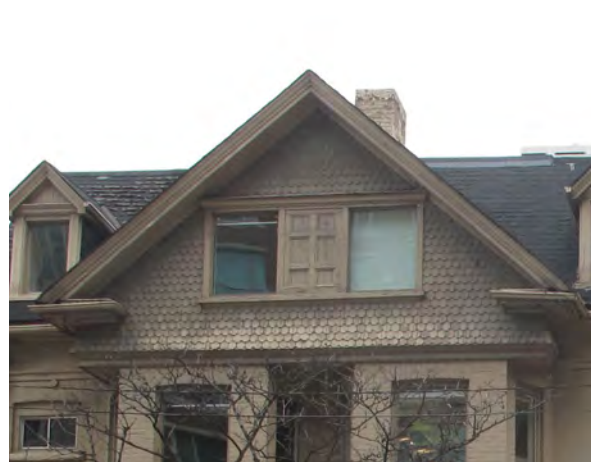
6. Example of general deterioration of decorative shake in gable on northern building (ERA, 2016).
