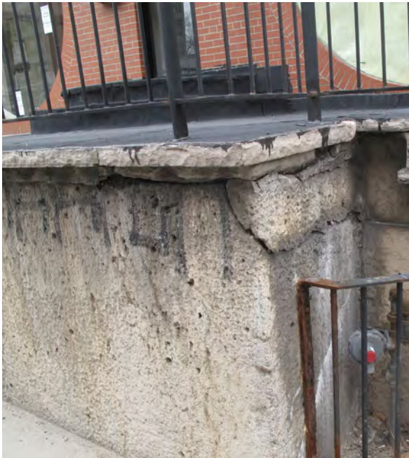
12. Partial view of porch in front of 45 Avenue Road, detail of tar sheets and deteriorating concrete (ERA, 2016).
