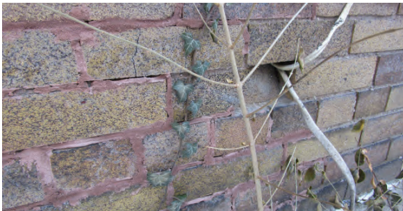
Detail showing masonry in poor condition (ERA, 2018).
