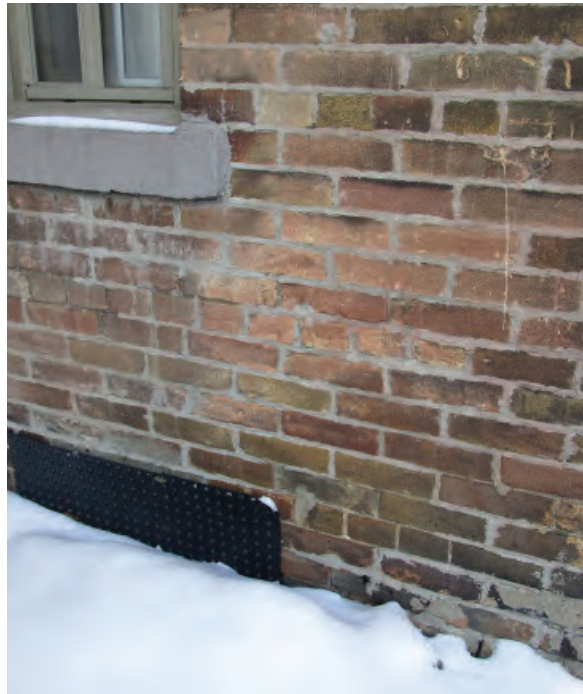
Detail showing poorly executed previous masonry repairs using unsympathetic cementitious mortar (ERA, 2018).
