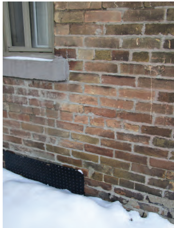
Detail showing poorly executed previous masonry repairs using unsympathetic cementitious mortar (ERA, 2018).
