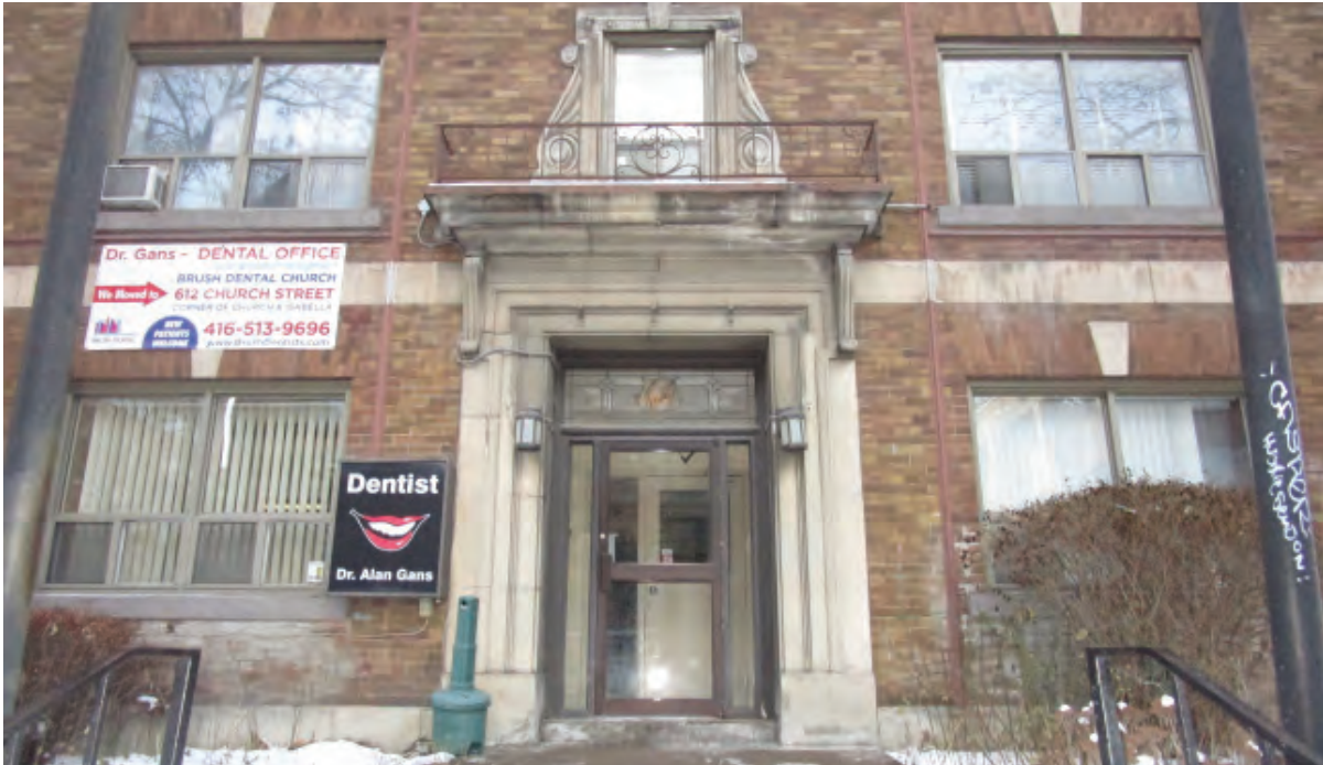
South elevation showing deterioration of cast-stone trim and staining of masonry under windows (ERA, 2018).
