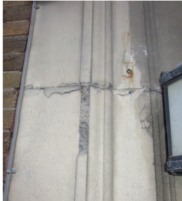
Detail showing deterioration of cast-stone door surround (ERA, 2018).
