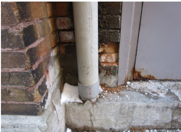
Detail showing spalled masonry near grade due to salt damage (ERA, 2018).
