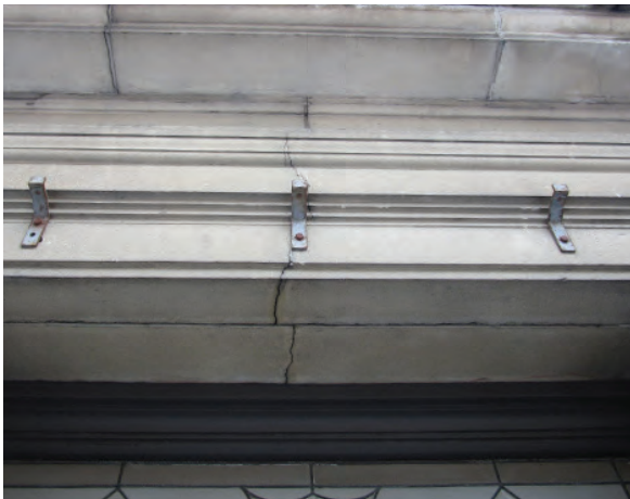
Detail showing evidence of settlement in building (ERA, 2018).
