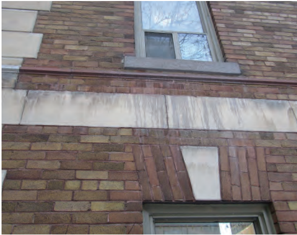
Detail showing environmental staining -- typical (ERA, 2018).
